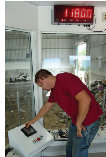
The BlokPak 3000 control station features a color touch-screen interface. This installation also has an integrated weighing system that displays the accumulating weight on-screen and on overhead monitors while the waste is being processed.
